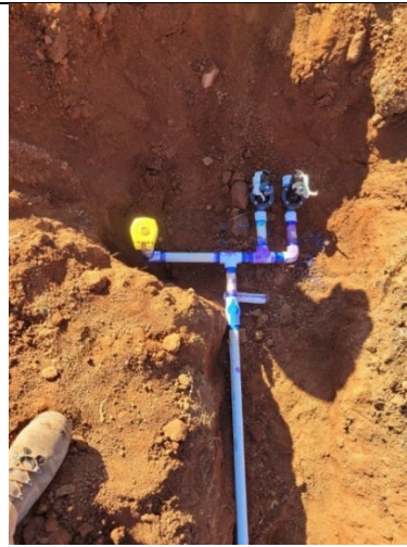
Figure 4. New irrigation at Nobel Park.
