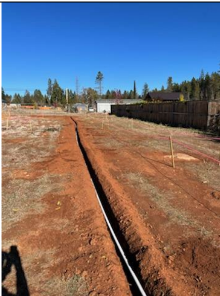
Figure 5. New irrigation at Nobel Park.
