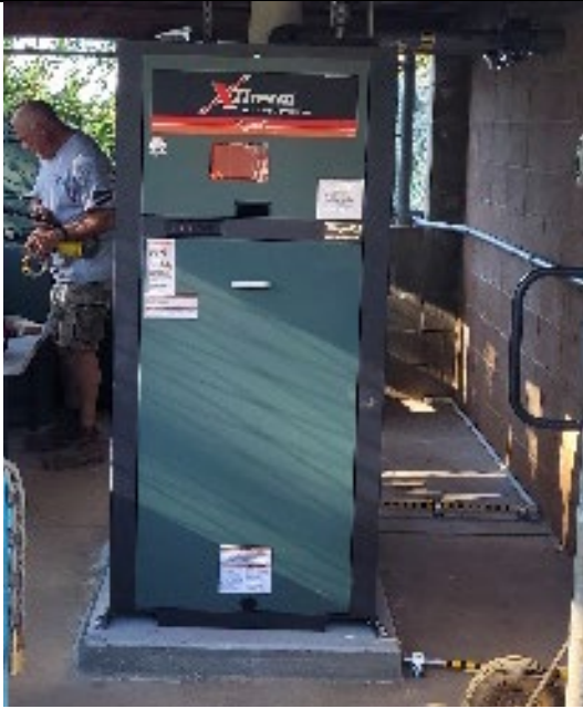
Figure 5. New boiler is installed and ready for those cold months.
