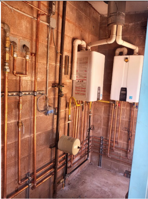
Figure 9. New tankless water heater at the pool.
