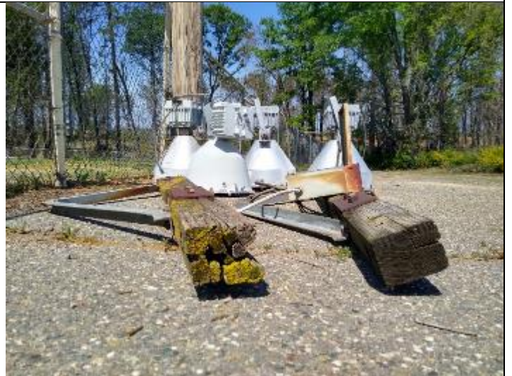
Figure 8. Cross-arms and fixtures on the ground
