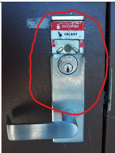
Figure 3. Restroom lock replaced due to vandalism.
