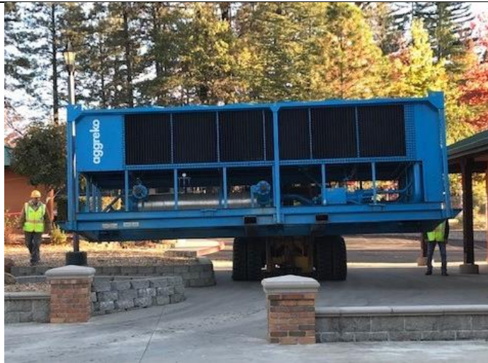
Figure 1. The Chiller has arrived! Kudos to Ray Lockridge on the forklift operation.
