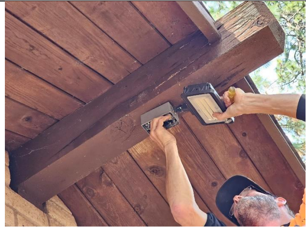
Figure 8. After the recent storm there were several lights that needed fixing at Bille Park.
