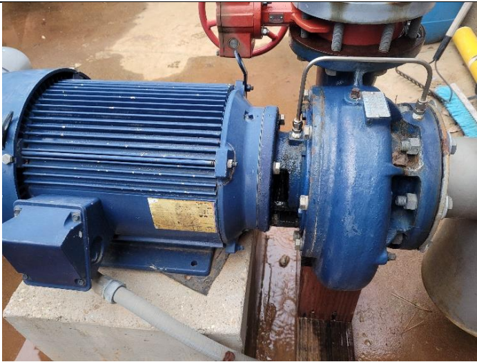
Figure 5. The pool pump getting a much-needed tune up.
