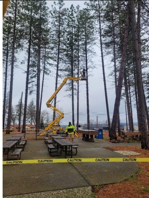
Figure 14. Maintenance worked on clearing the broken tree to avoid accidents and further broken trees.
