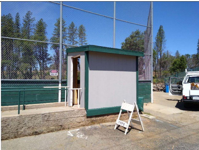
Figure 11. The finished score booth. Now it just needs the re installation of electricity.
