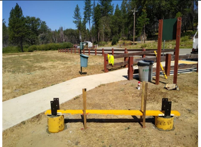
Figure 20. Shout out to maintenance for installing cement footings for eagle scout project.
