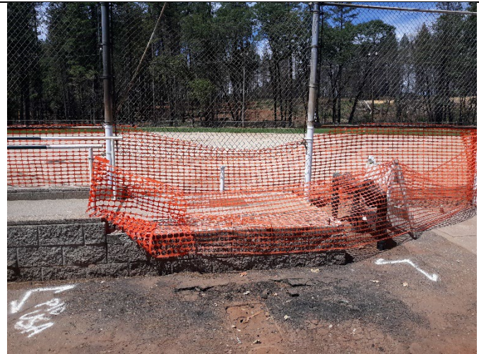
Figure 10. The beginning stages of the new score booth at Moore Rd. Ballpark.
