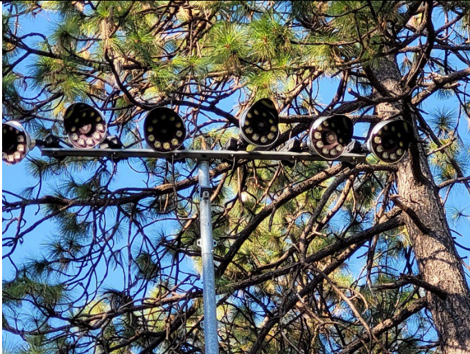
Figure 11. The replaced light at the ballpark.
