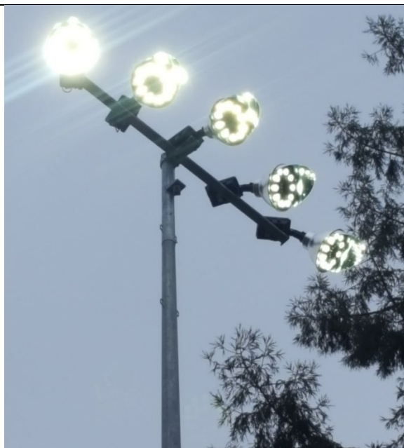
Figure 8. New LED lighting fixtures at Moore Rd Park
