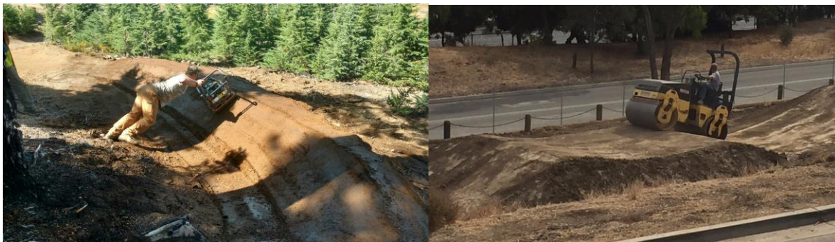
Compacting a berm turn with a vibrating plate compactor. Compacting the large dual slalom features with a roller compactor.
