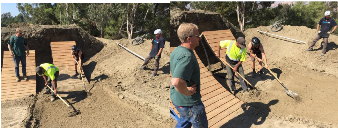
Condition soil with rake or shovel, chop up clods, then smooth, shape and compact.
