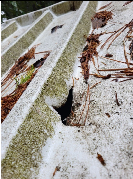
Figure 11. The roof to one of the Porta Pottys at Paradise Lake needed repairing (Before).
