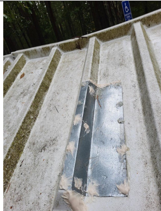
Figure 12. The roof to one of the Porta Pottys at Paradise Lake needed repairing (After).
