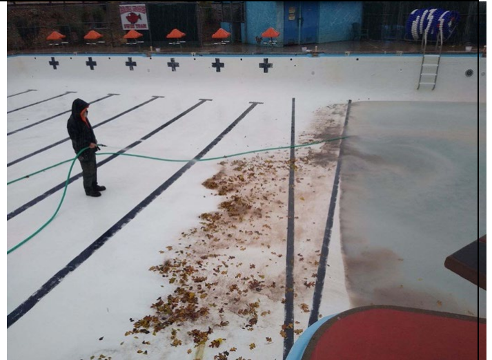
Figure 6. Maintenance staff spraying out the dirt from the bottom of the pool.
