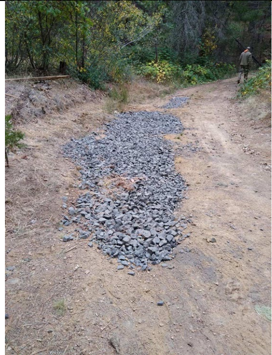
Figure 8. A large rut on the Paradise Lake Trail (After).
